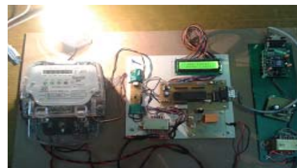
Fig.8: AMR Transmitter unit when the load is ON
